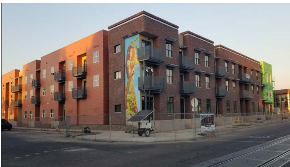
This October photo shows The Lofts at Fort Visalia in the final stage of construction on the northeast corner of Garden and Oak streets.
